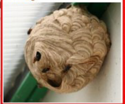
Secondary nest in a building
